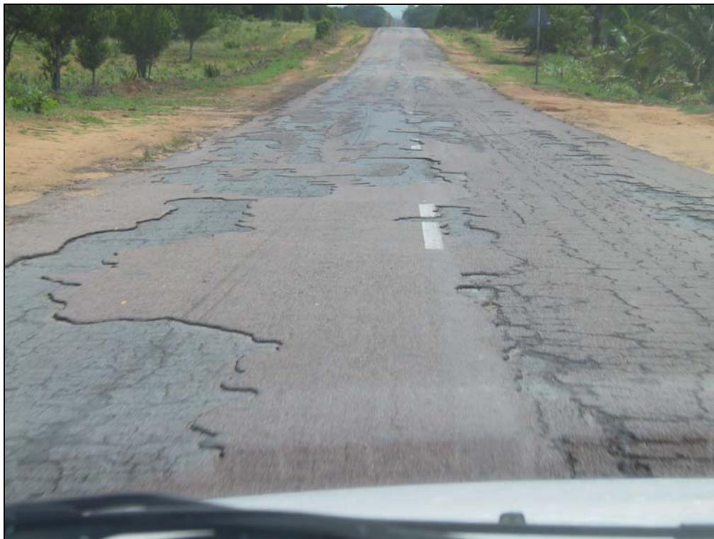
Figure 2-3: Some sections of the EN1 lost the top tar layer and contain significant potholes.
