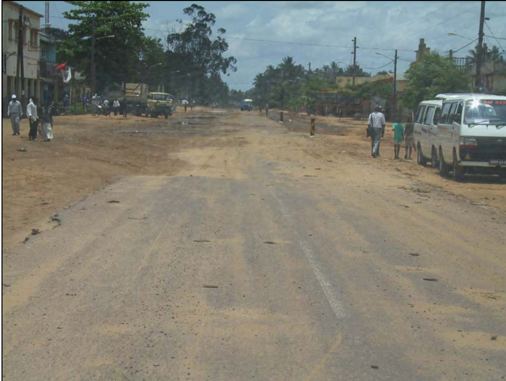
Figure 2-5: Many towns are characterised with bad water drainage due to the lack of storm water drainage systems. Potholes are not visible during intensive rain storms and are often filled with muddy water following the episode, making it difficult to identify.
