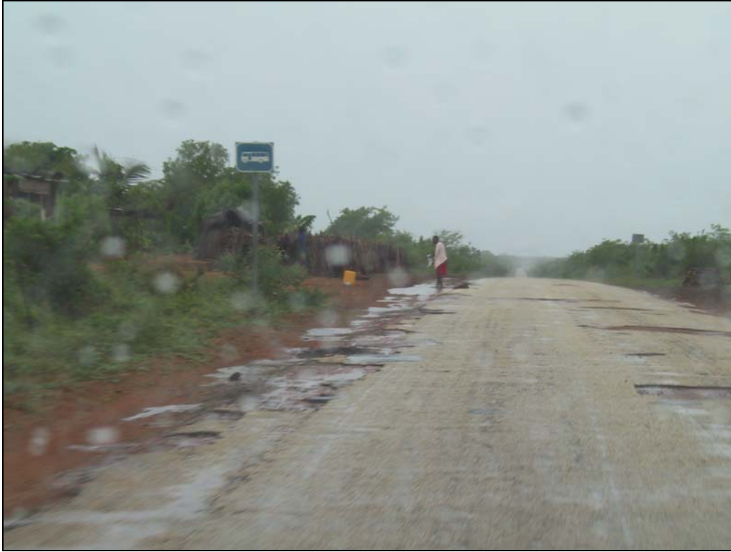
Figure 2-4: The road edge has in places significantly eroded away along the EN1.
